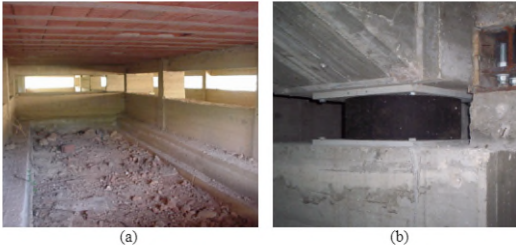
Figure 19: Squat columns in the original building before (a) and after (b) the insertion of the seismic insulators (After Caliò and Marletta [28]).
